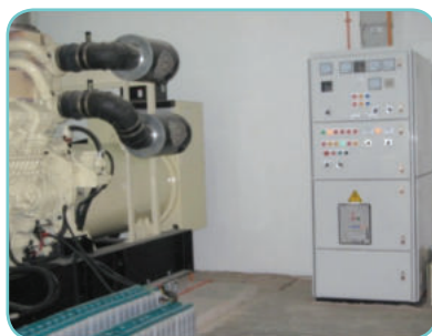
Naiktaraf kapasiti genset Hospital Melaka
